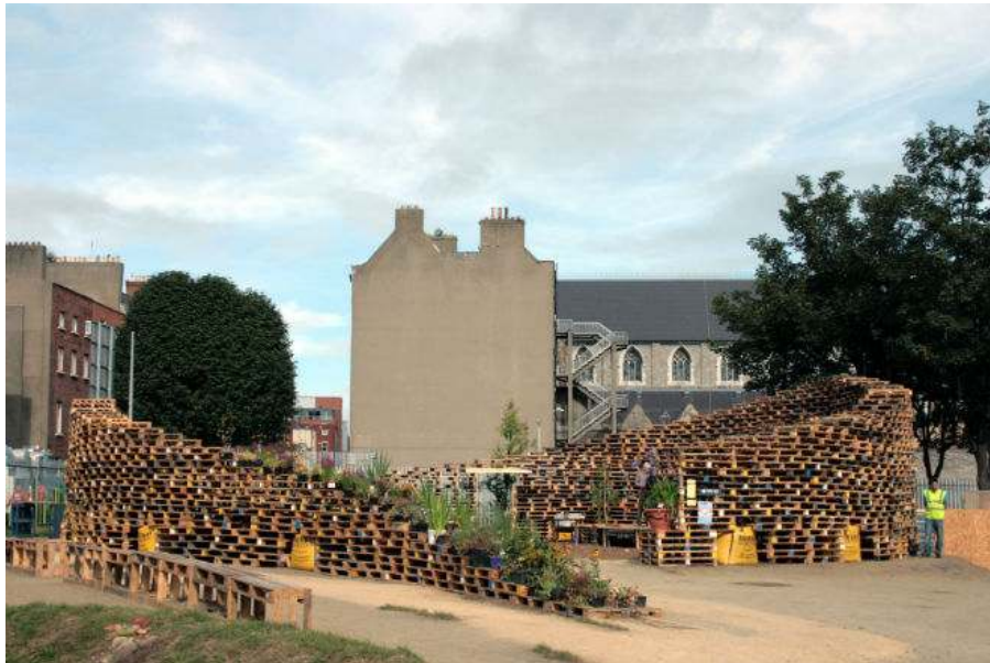
F16. Granby Park, Dublin by Upstart– Vacant site in the heart of the city revitalised by 500 volunteers for 4 weeks of art and performances 32
